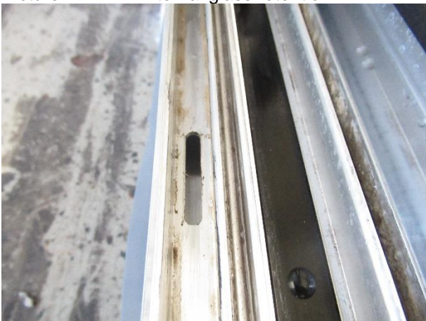
Picture 29 Drainage slot bottom track
